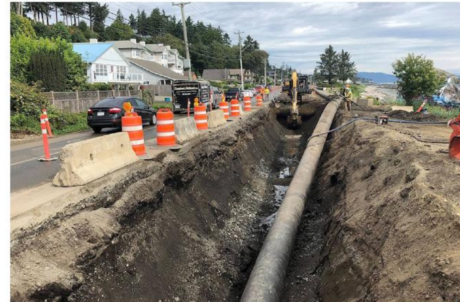
The Highway 19A construction project has wrapped up for the season after a midden was discovered near Rotary Beach Park. A midden is archeological evidence of past First Nations occupation in the area. Image provided
